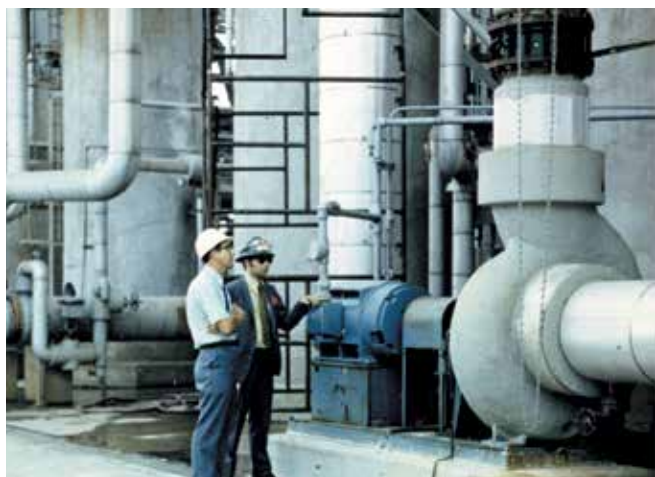
A 3175 installed in a major chemical plant.
